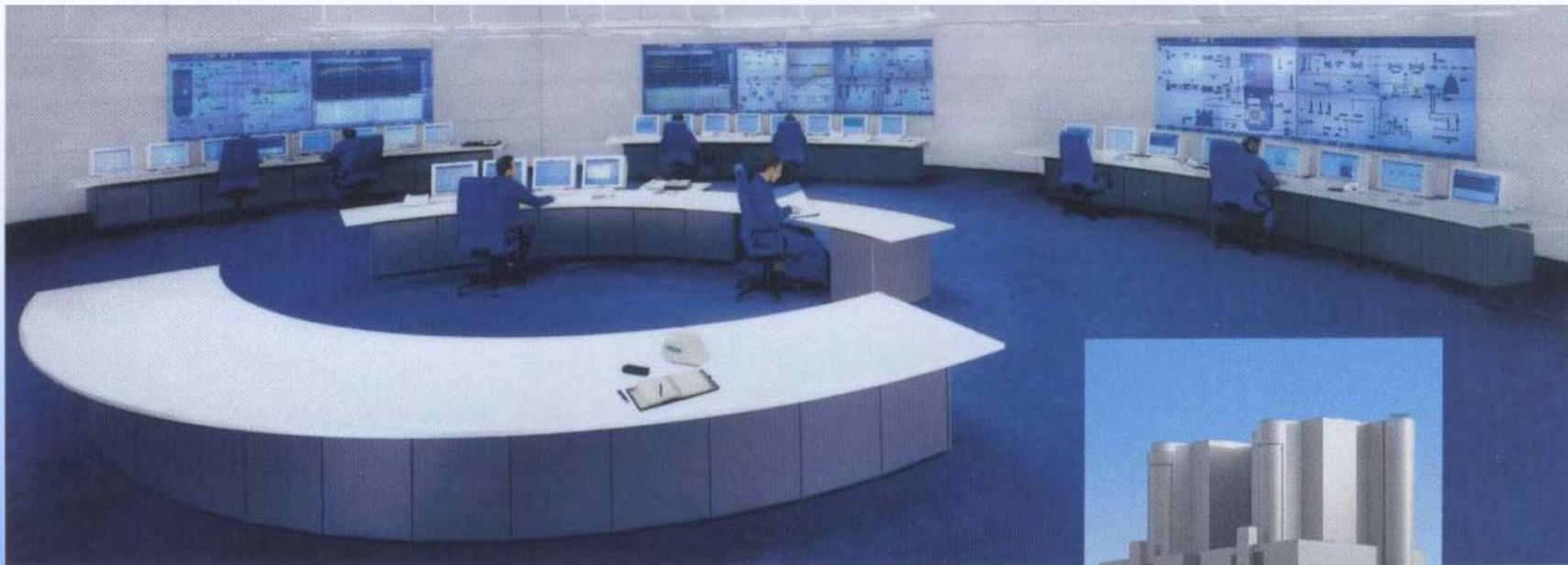
Control room implemented in Schwarze Pumpe, Germany
